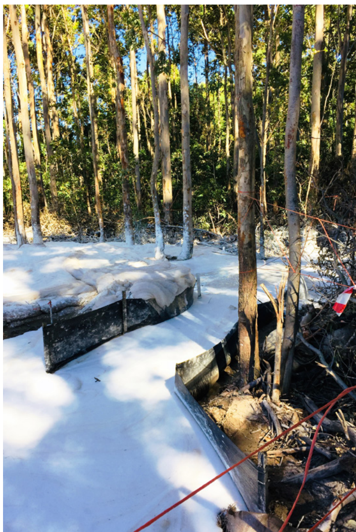
Drilling in process, with Rotofoam mix and fines spilling over sumps and silt traps.
